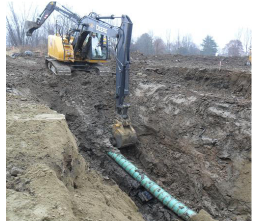
Clean up of the asbestos contaminated soil along the trail bed behind Wemelco Way (photo courtesy EPA)
