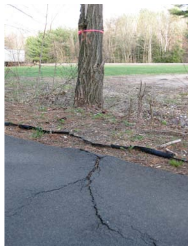
A tree that has been marked for removal due to root damage to the trail near South Street.
