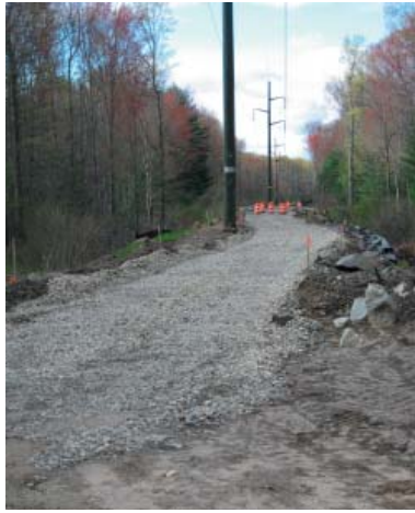
A gravel base has been laid just north of Lovefield St. but other parts of the new Manhan Rail Trail spur from Easthampton and Northampton have a base layer of pavement.
