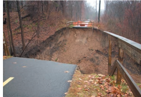
This house-sized sinkhole developed after an old railroad culvert collapsed near East Street last September pulling down the rail trail surface and fence along with it.
